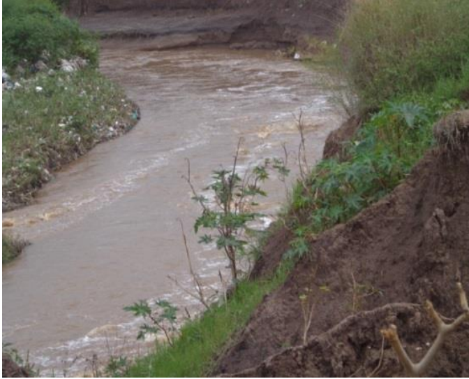
Figure 11. Undercutting of outer bank. Source: Monene 2014: Photos taken on 17/12/2013 during wet season) and 5/9/2013 during dry season.
