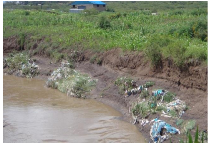
Figure 10. Basal Cleanout of the outer bank. Monene, 2014: Photographs were taken near Kangundo Road Bridge on 28/12/2012.
