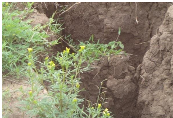
Figure 7. Unstable outer bank showing cracks. Monene, 2014: Photographs were taken 10 m downstream of Kangundo Road Bridge on 17/12/2013.
