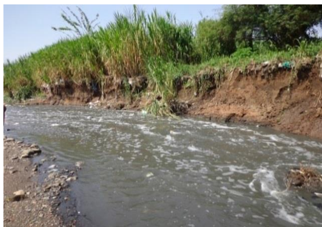
Figure 6. Collapsing of banks. Source: Monene, 2014: Pictures taken on 17/12/13 and 5/9/13.
